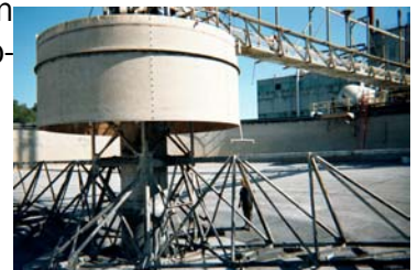
Coated Fill Tube after 6 Years Service
