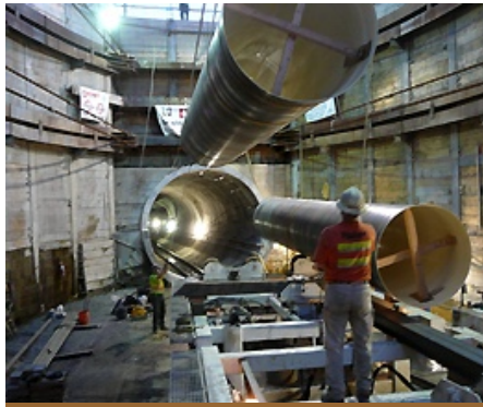
Service Pipe Entering the Tunnel
