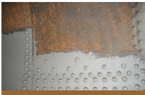
Deteriorating substrate during mechanical blasting
