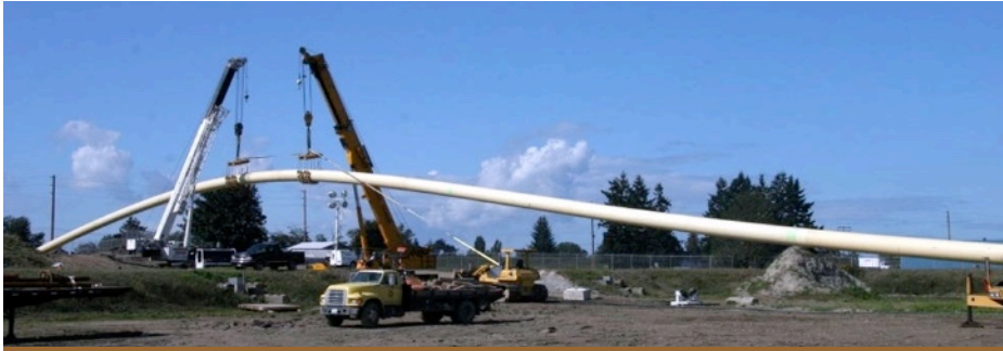
Crews Strung Preassembled Pipe Lengths Through the Air to Feed into the Drill Pit Hole
